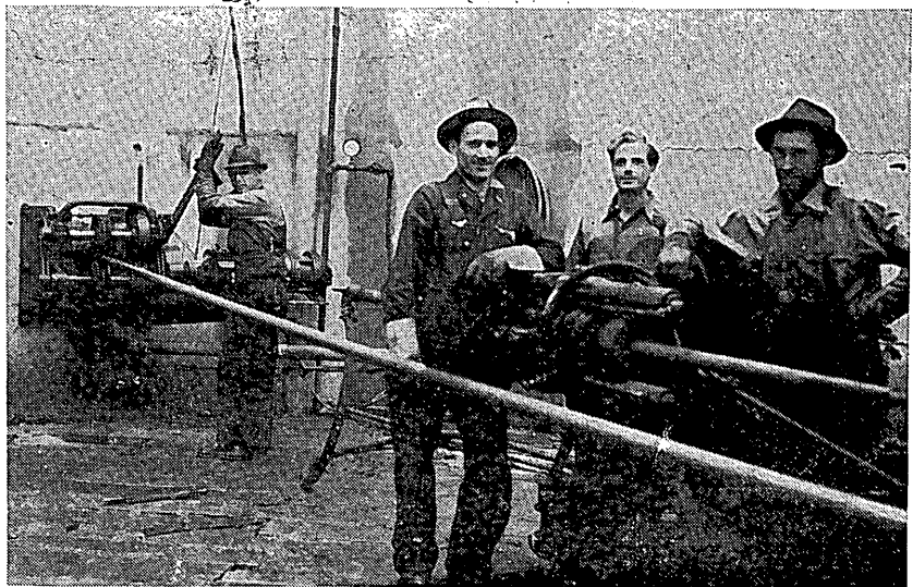
"Drilling two wells at a time". Pulling 50 feet of core from one well while running another set of tools and the drill rods into the opposite well. This is done by the newly developed "rod puller" which moves the tools at the rate of 100 feet per minute. Drill rods are not disconnected until both wells have been drilled to the desired length. Drilling machine is moved back (hydraulically) while tools are being moved. Compressed air motors are recommended as the best power for all machines in the work chamber.
